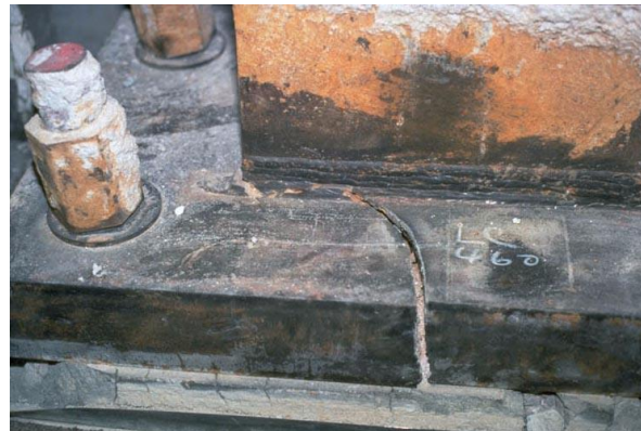
Fig. 1-13. Fractura en una placa de base de columna de una estructura de pórtico arriostrado ( Earthquake Engineering Research Institute, Slides on the January 17, 1994, Northridge Earthquake, Set I: An Overview ).
